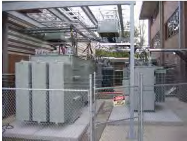
12.5 kV and 4.16 kV transformers
