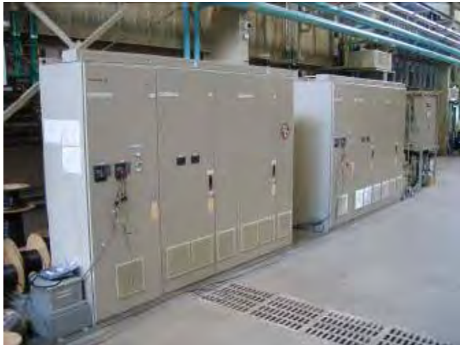
2 x 8 MVA / 5 MW variable speed drives
