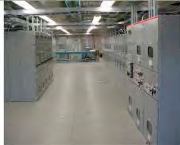
12.5 kV and 4.16 kV switchgear
